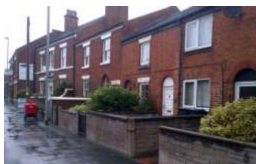
Effect of traditional brick walling undermined by use of modern 'Artstone' in foreground
