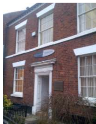
6 over 6 sash windows in this listed Georgian property. Also not the panelled door surround with pediment and dentil moulding to fascia board
